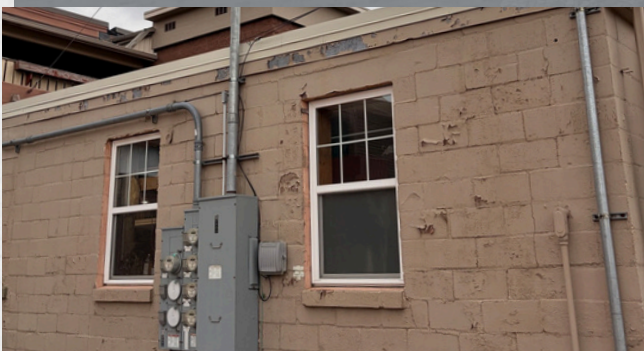
Before: Exposed electrical pipes and peeling paint
