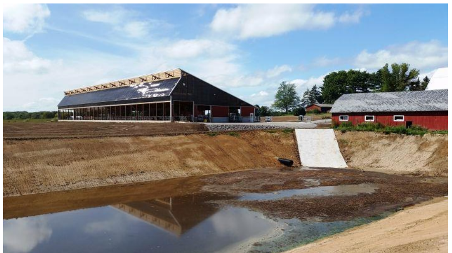
clay lined waste storage facility
